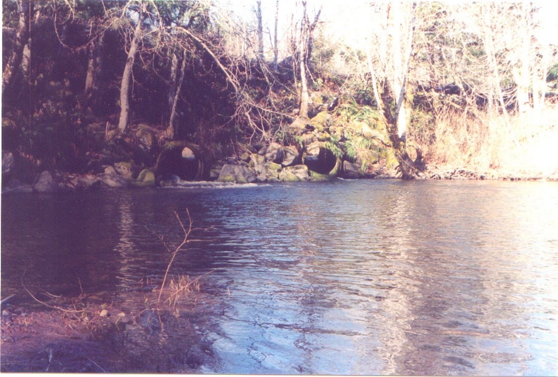
Figure 16. Culverts under the U.S. Navy railroad crossing on Sherwood Creek (RM 6.8) prior to replacement with a bridge in fall of 2002. Photo courtesy of the Allyn Salmon Enhancement Group.
