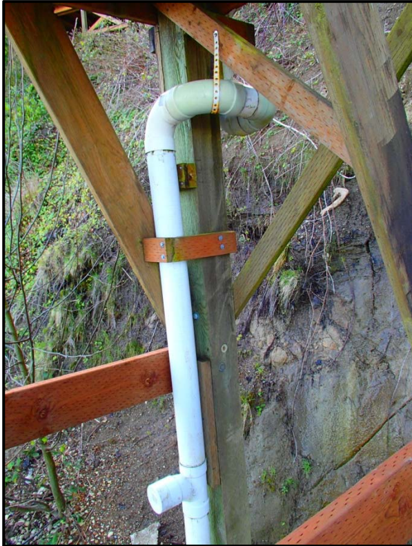
Above: a well-secured, solid drain pipe carries water down the face of a bluff to a safe outlet near the base of the slope. A system like this is easy to clean and monitor for leaks.
