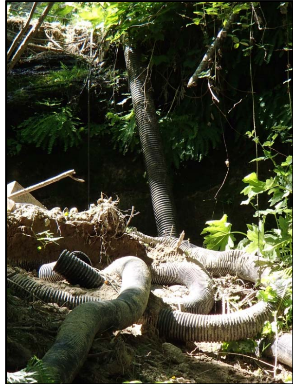
Above: an example of a failed drainage system associated with a landslide. Poorly-secured pipe connections, undersized drainage pipes, or leaks in conveyance pipes can compromise the integrity of drainage systems. Good design and regular monitoring can help identify issues and prevent failures.
