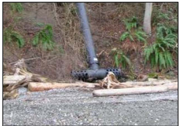
Above: a pipe with a “diffuser tee” that outlets water near the base of a slope. The diffuser is attached to the end of the pipe to slow the water down and decrease its energy as it exits, thus preventing beach erosion.
