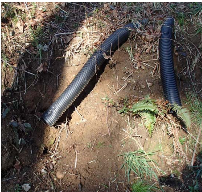
Above: a problematic drainage pipe that releases water on the face of a slope rather than at the base. The water does not slow down as it leaves the pipes, which results in scouring and bare soil. The slope is beginning to erode and will only get worse without improvements.
