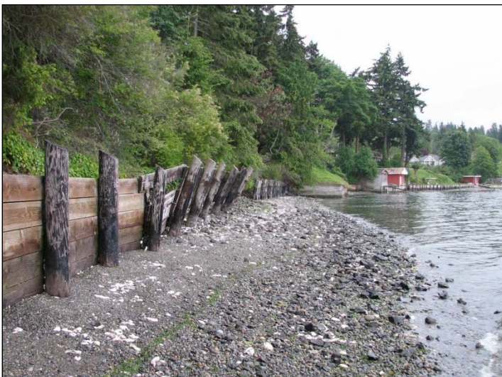
BEFORE: A failing bulkhead serving no practical purpose.
